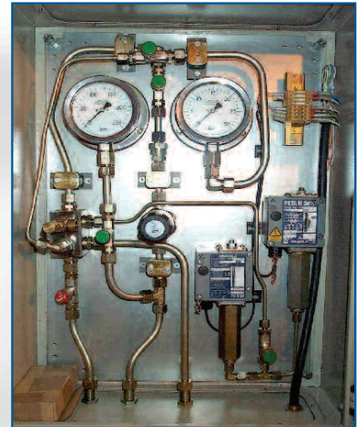
New Control System
